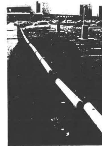
Photograph 7 The slide in the parking lot of the Boathouse Restaurant has severely damaged the concrete walk along the southern side of the parking lot and extends 8 feet (plus or minus) into the asphalt pavement of the lot.
